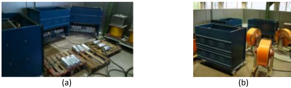
Figure 5.42. Passive loads with capacitors mounted (a) and with inductors mounted (b).
