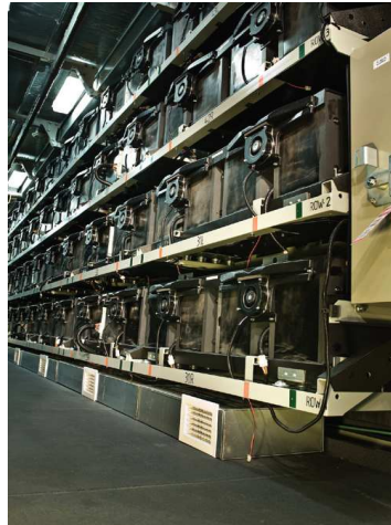
Figure 14: Large Li-ion battery facility for frequency regulation.
