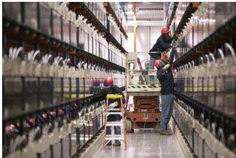
Figure 10: Biggest BESS in the world in Fairbanks, Alaska, USA.
