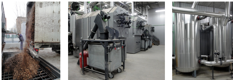
Figure 6. New biomass boiler room and silo
