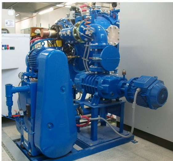
Figure 7.4. Rotary piston pump H149 (left) and mechanical booster MB43 pump (right).
