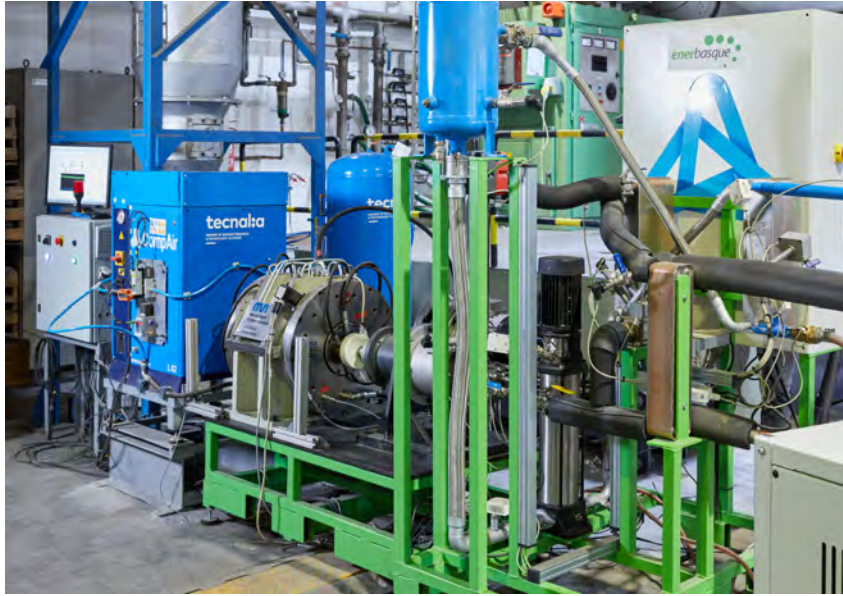
Figure D.1: RECUWASTE solution. The manufactured and tested WHRS.
