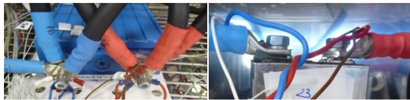
Figure A-15. Prismatic cells connection
